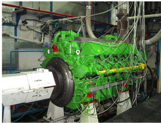
Fig2. D87 dual fuel engine in test cell
